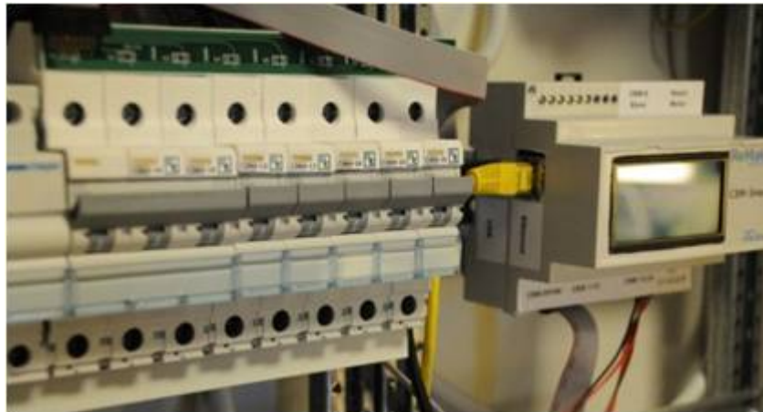
Image 3: A typical hardware installation. A row of CBMs with a SmartBar on top (partly visible) and a SmartGate to the right.
